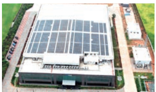
Makino India Private Limited. (Coimbatore, India) Estimated power generation: 684,000 kWh/year (power generation started on March 31, 2024)
